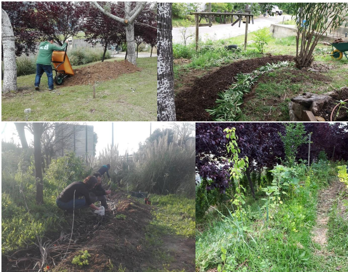
Figure 45 Swale building in PermaLab (2018). Lines are formed by accumulating organic matter at the same level on a slope (upper left picture), acting as an obstacle to water runoff. In these lines, there is an upstream depression (the swale) where more coarse organic matter is accumulated to incorporate biomass into the soil (upper right picture). Plants are planted at the crest of the 'mound' (bottom left and bottom right pictures).
